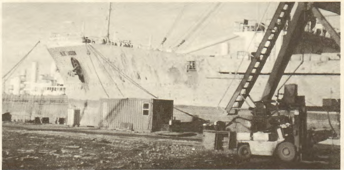
When the Blue Lagoon was arrested in the port of Detroit, corrosion and rust on the hull were evident.
