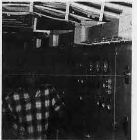
Chief Electrician Randall Lawson holds a steady hand on the Oakland's power panel as the vessel heads towards its port.
