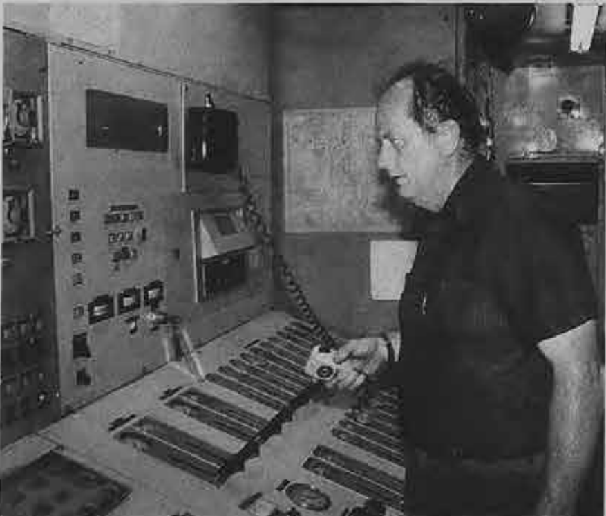
Pumpman William Dooling keeps an eye on the ballast tank gauges.
