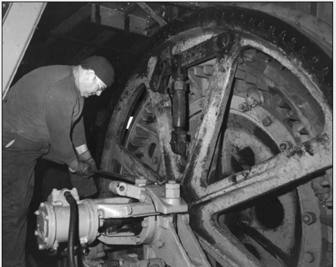
Deckhand John Monaco tightens the bearing cap of the main drive gear on a Great Lakes Dredge and Dock dredge during Great Leaks fit out in early 1979.
