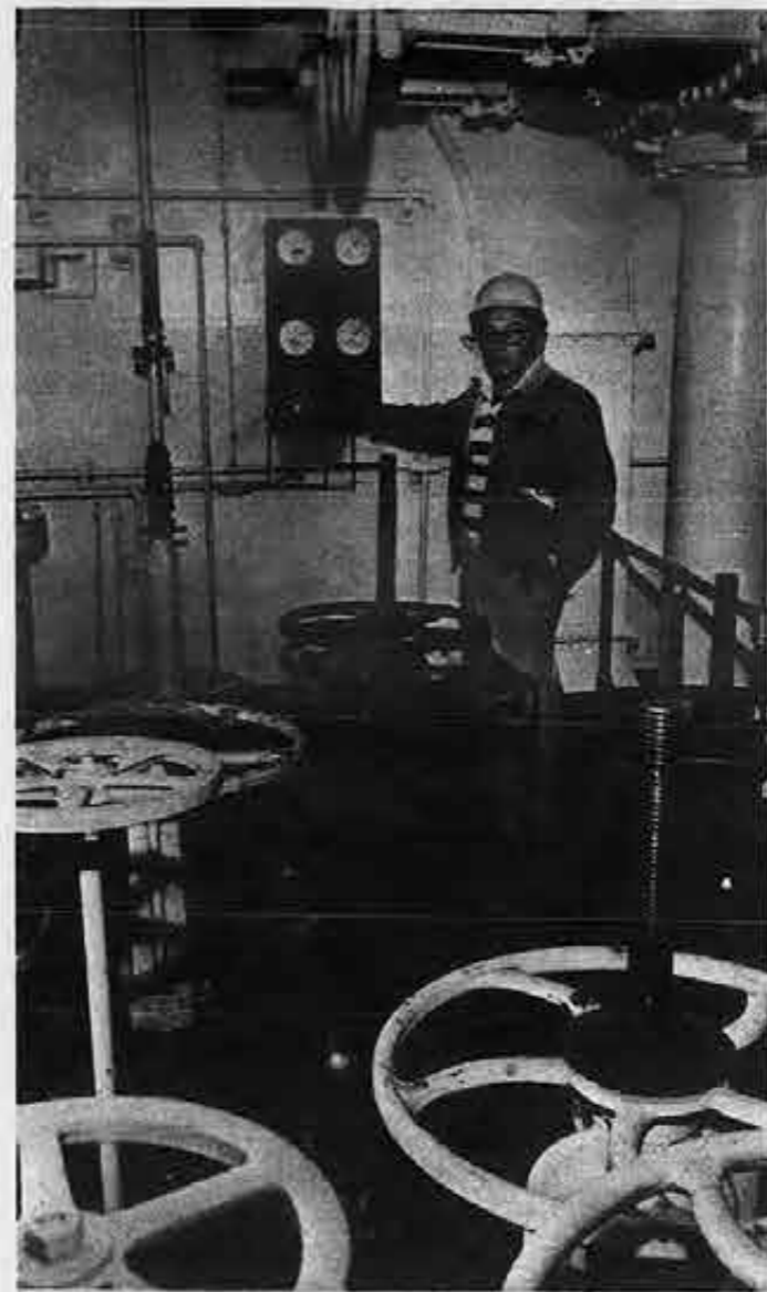
QMED/Pumpman Joseph Arpino checks a gauge in the pumproom.
