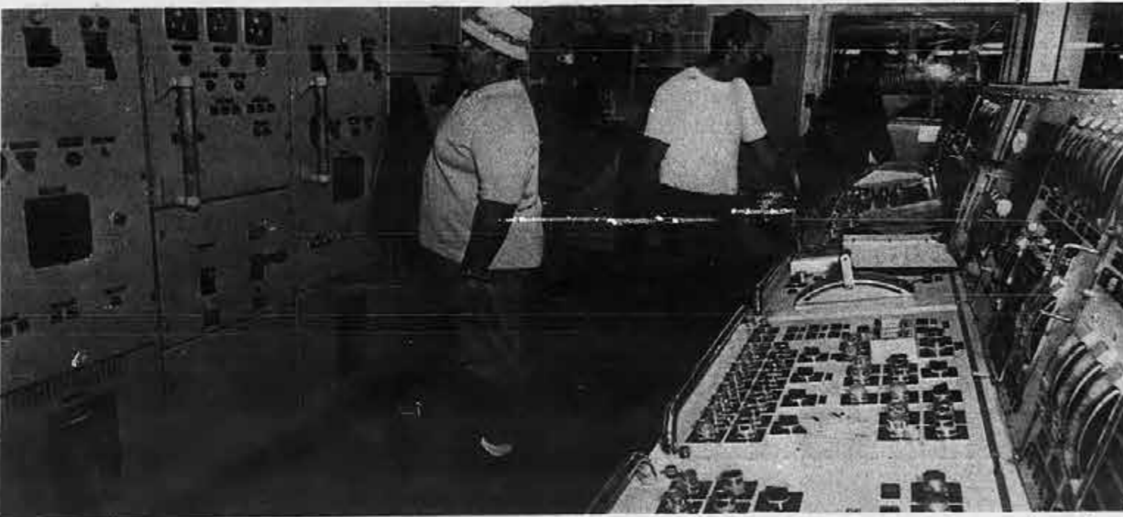
Piney Point QMED grads Joseph McGauley (left), Mitchell Hill (center) and Jack Davis check out the vessel's main engine control panel.
