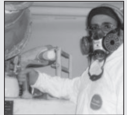
GVA Mohamed Mohamed sprays a new coat of paint on the SS Cape Intrepid.
