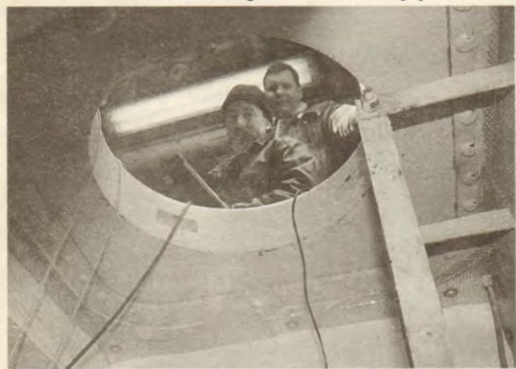
Confined-space safety and rescue training, part of the school's tanker operation/safety course, is designed to bolster members' skills.
