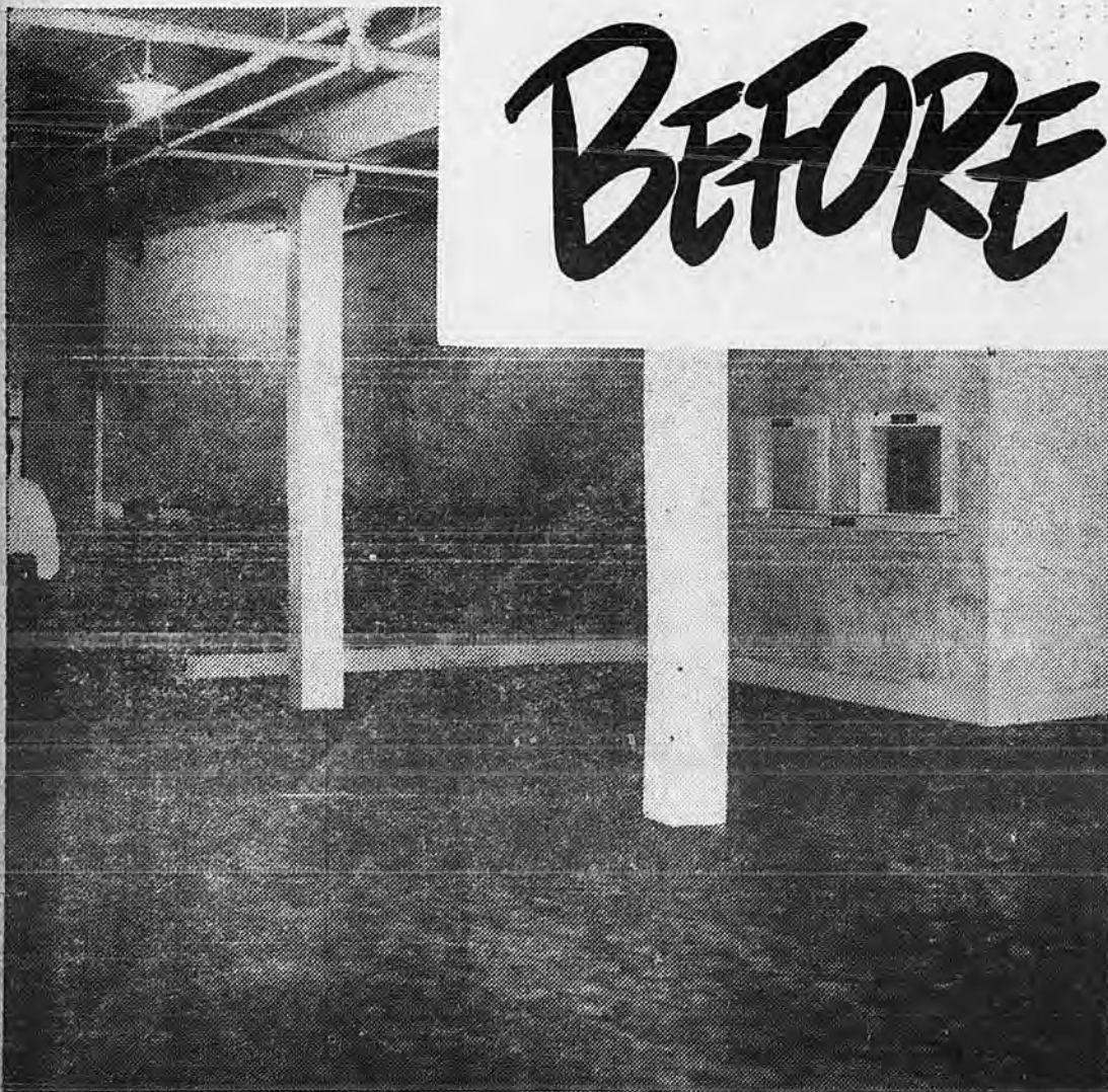
Compare this scene with the ones above before the Hall was readied for occupancy. Now all members can be accommodated at meetings, instead of only half those attending. Not another union hall in the South can compare with the Seafarers Hall in New Orleans.
