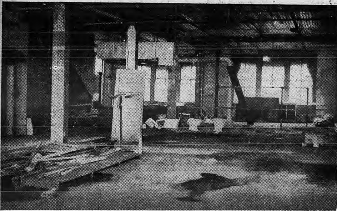
It took hard work to get the new Hall in ship-shape condition. Starting with the filthy and dilapidated interior (above) and handicapped by a fire which further messed up things, within a few months SIU men, working under the supervision of Frenchy Michelet, made the changes and improvements which appear below.
