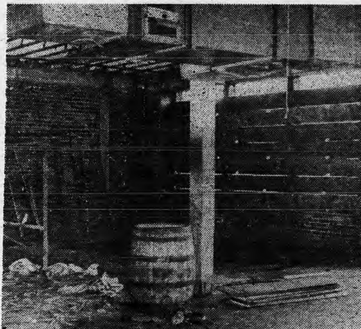
The fire damage was quickly cleared away, and then the job of renovating the Third Deck was gotten under way. Insurance paid for the damage and, with willing hands to do the work, the wrecked structure soon became first class.
