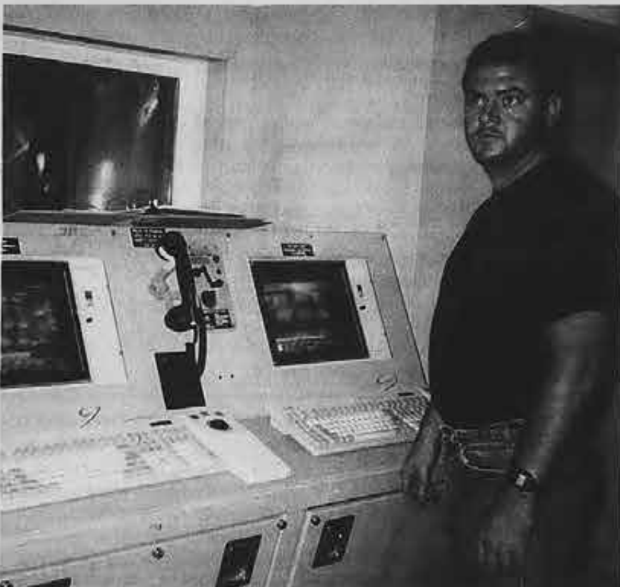
QMED Troy Robin looks over the computer monitors in the state-of-the-art engine room aboard the Sulphur Enterprise .
