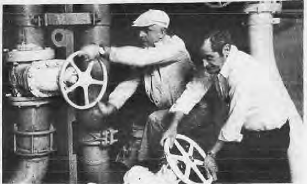
Daniel O'Rourke and Stephen Homka work in the barge's pumproom to line up the cargo transfer system.
