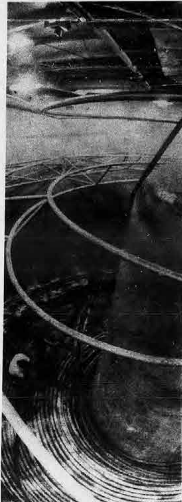
From the huge tank on the vessel some of her 1,000 nautical miles of cable go above deck to be laid in the ocean.
