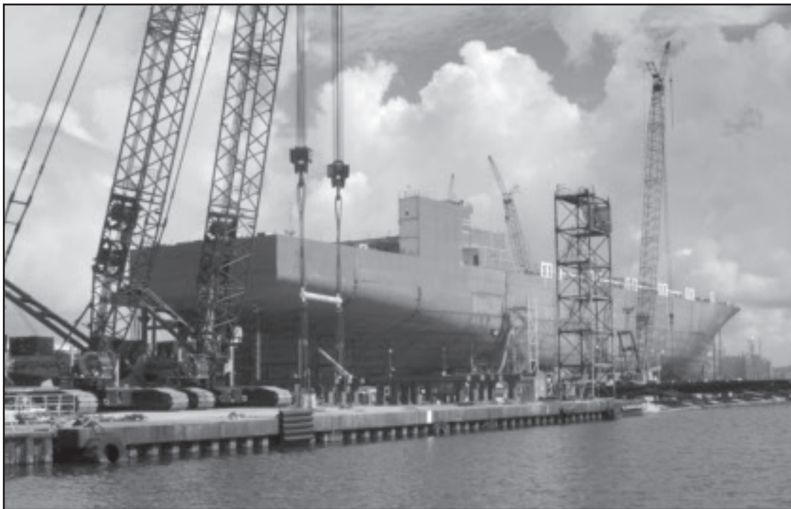
Construction continues on the El Coquí , which will be crewed by SIU members. (Photo by Brian Moran)
