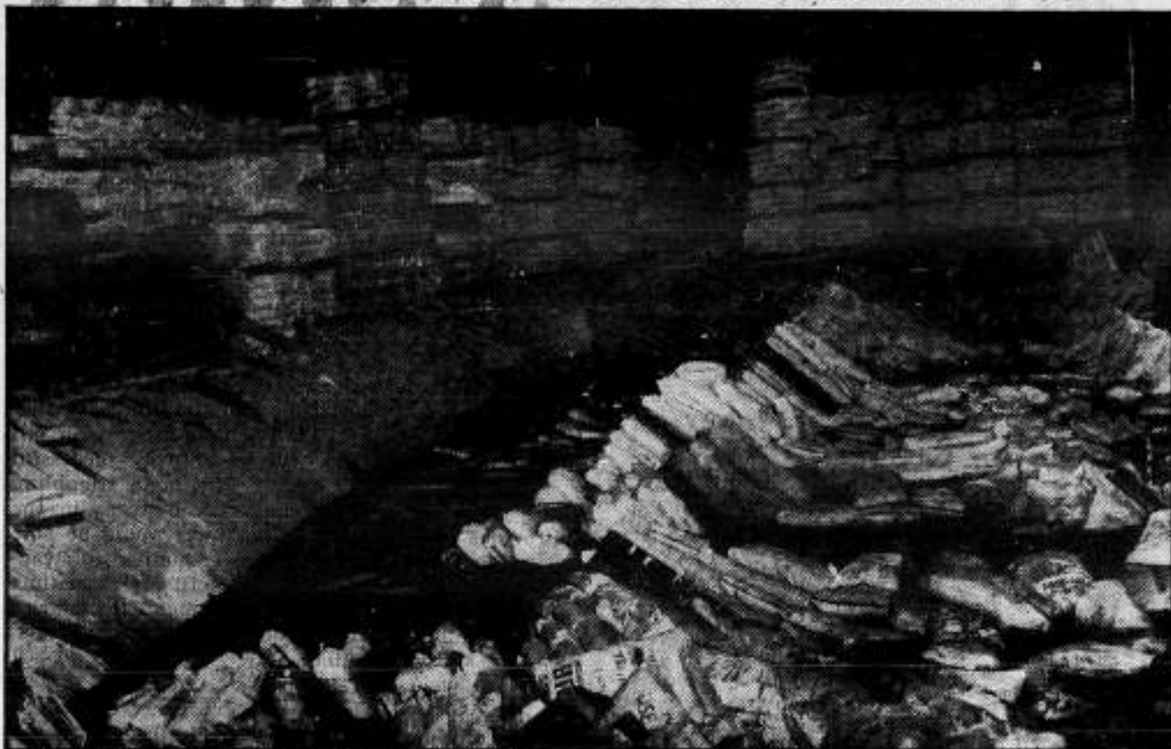
Rotting timbers of Huron Street storage pier in Brooklyn gave way and dropped this 1,750,000-pound cargo of tapioca into the East River. Although no one was injured, AFL Longshoremen were called off the job of moving the cargo when danger arose the whole structure might collapse.
