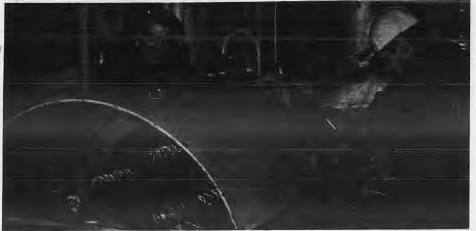
Oilers Frank McGuire, left, and Dick Hogut work on the service generator aboard the McKee Sons .
