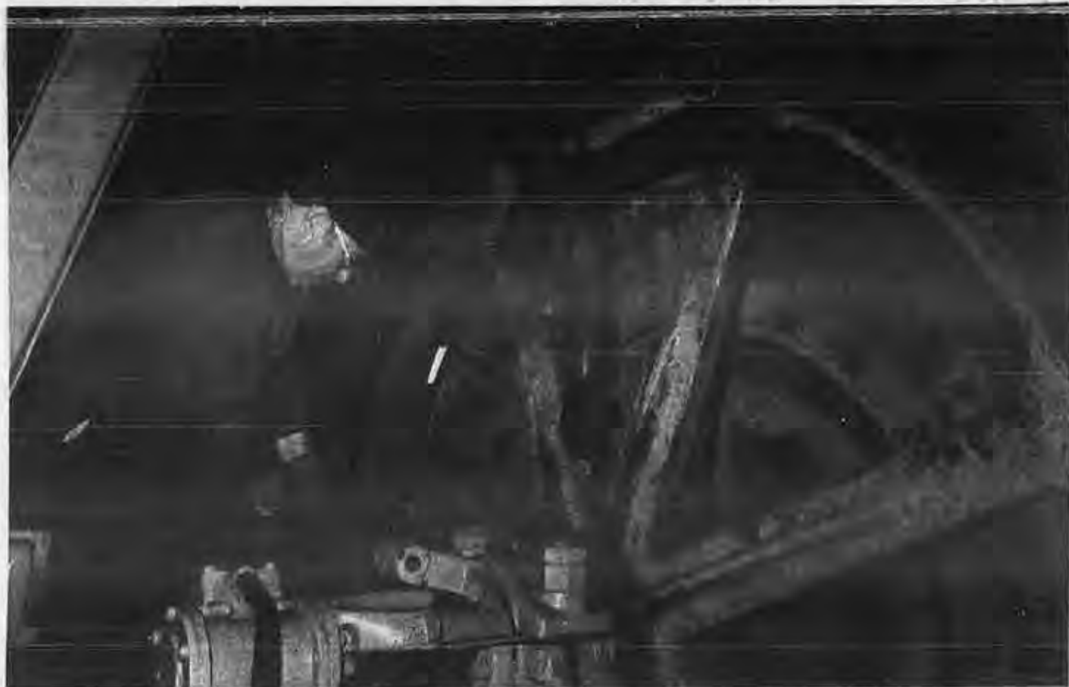
John Monaco, deckhand, tightens the bearing cap of the main drive gear on a Great Lakes Dredge and Dock dredge.
