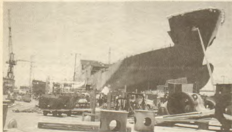
Future job opportunities for Seafarers are evident at NASSCO, where construction of another Watson -class ship is well under way.
