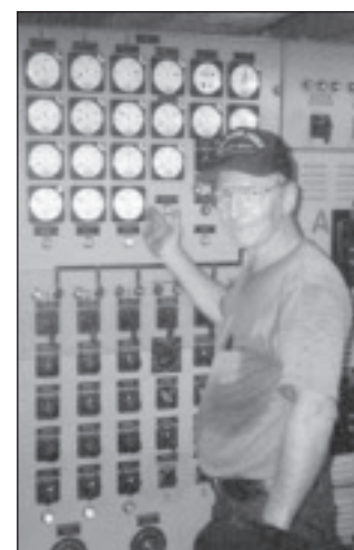
Electrician Bruce Callaghan monitors the gauges in the engine room.
