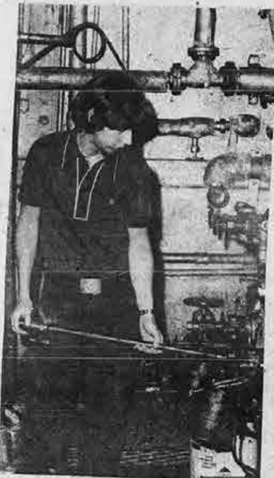
Upgrader Craig Spencer works in the Lundeborg School's engine room as part of his on-the-job training for FOWT.
