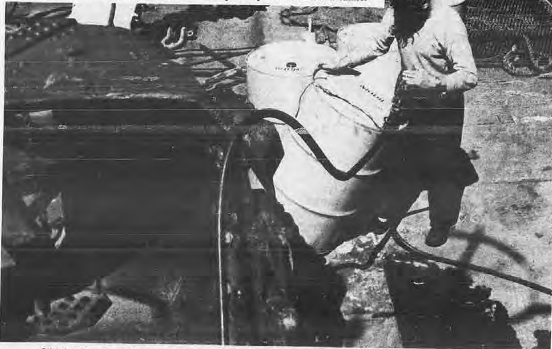
SIU deckhand Jim Burns working on the Dunbar & Sullivan Co. tug Sachem during fit out in Cleveland.
