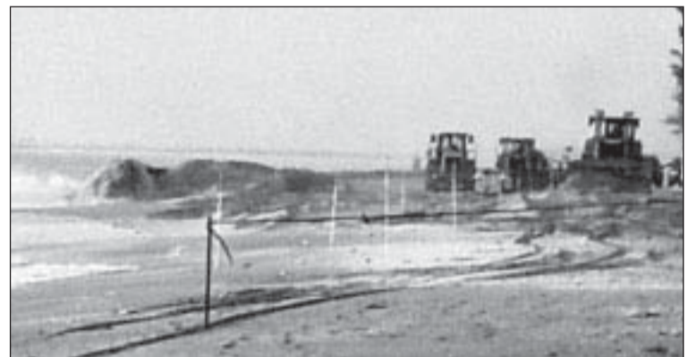
Sand is pumped ashore to rebuild the beach line on Captiva Island.
