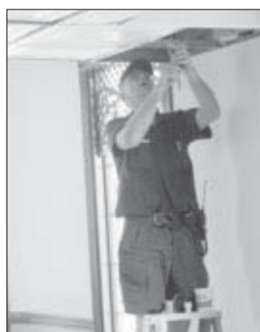
Chief Engineer Bob Buttmer adjusts the air conditioning.
