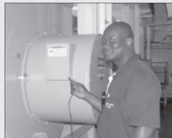
Electrician Ousmane Ka performs preventive maintenance on the generator.
