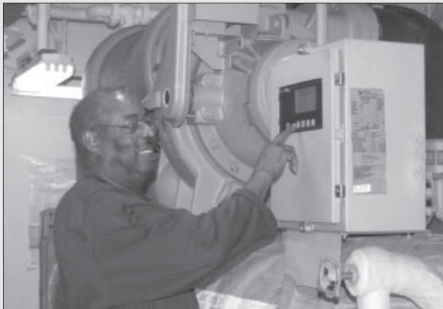
QMED Rutland Gale checks readings on the #2 A/C chiller.
