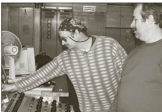
QMED Bob Oppel (left) and 3rd Asst. Engineer Mike Novak, an SIU hawsepiper, check the auxiliary diesel generators on the Cape Wrath .
