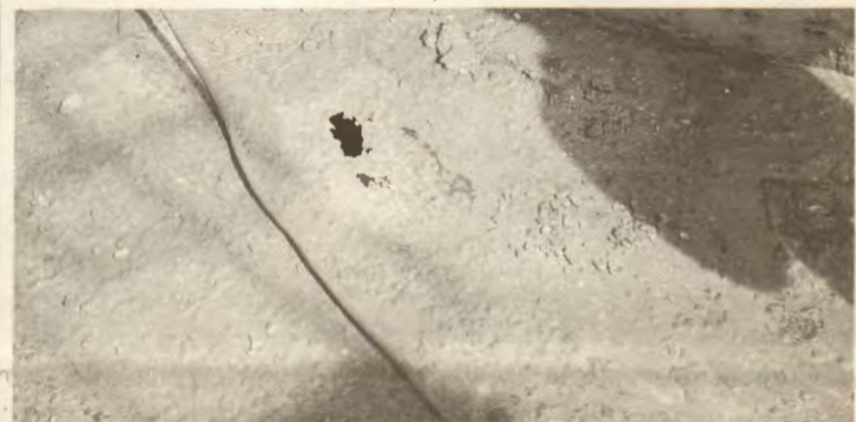
In some spots, the vessel's deck was completely rusted through.
