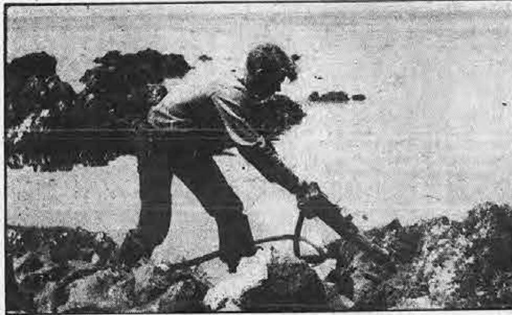
Pneumatic drills proved useful for cutting into rock ledges surrounding ship and gripping it to shore. Refloating operation took just one month before the San Mateo slid back into water.
