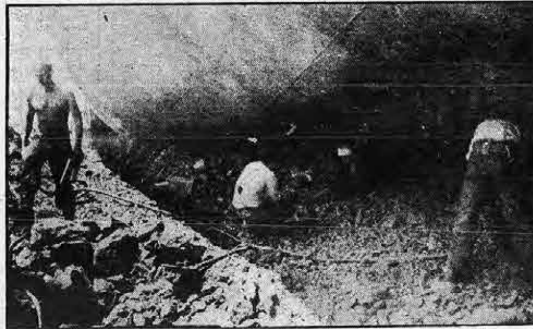
Holes were drilled into rock to place charges for blasting. Rock had to be removed from under the forepart of the vessel and also from places where it had cut through the ship's bottom.
