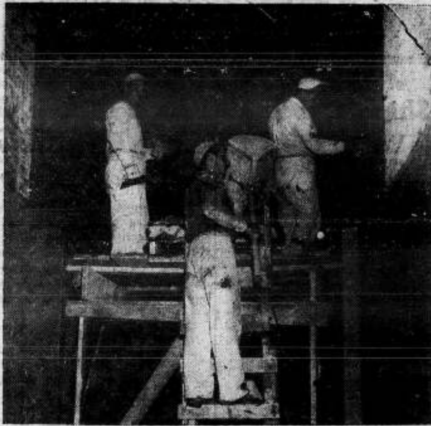
Union plasterers are shown at work on the second floor corridor of the A&G District's new Headquarters-New York building. As work continues on the structure, Seafarers are looking forward to its official opening, tentatively scheduled for some time in the summer. The new building is located on 4th Avenue, between 20th and 21st Streets in Brooklyn and is two blocks from the Prospect Avenue station of the BMT-4th Avenue local subway line.
