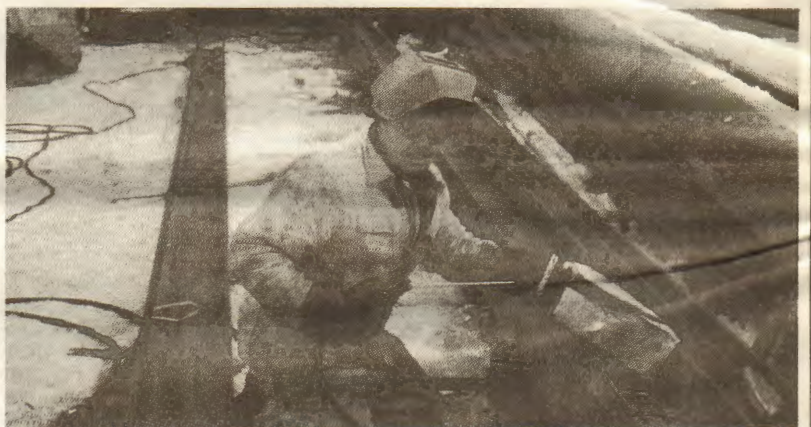
Using an angle iron to weld a lift support is Seafarer Bud Cropek.
