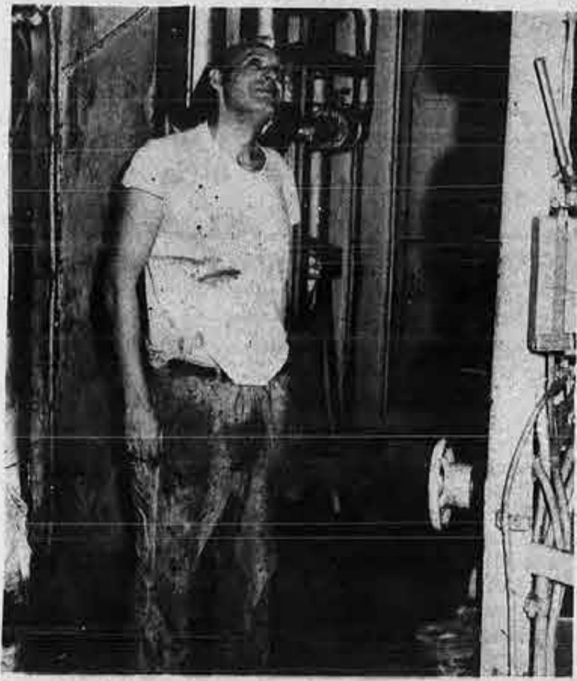
Fireman/Watertender Marcel Romano checks the water level in the Aleutian's boiler.
