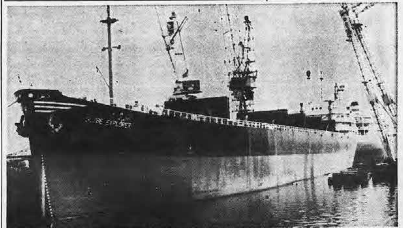
With her new stern section installed, the Globe Explorer , which was damaged by fire last year, is presently undergoing installation of new piping and wiring. Completion of the extensive reconstruction job is expected to take a couple of months.
