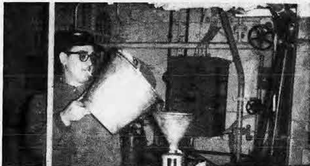
Oiler John Bailey starts oil purifying process on the steamer Paul Townsend to clear water accumulation and strain out impurities from below-decks machinery that have been idle all winter.
