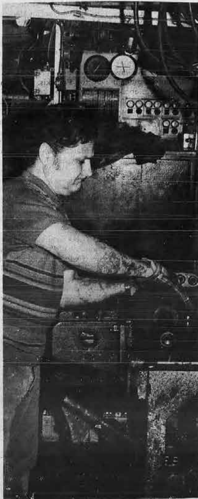
Fireman W. Cachola, also serving as department delegate, tends to duties in ship's engine room.
