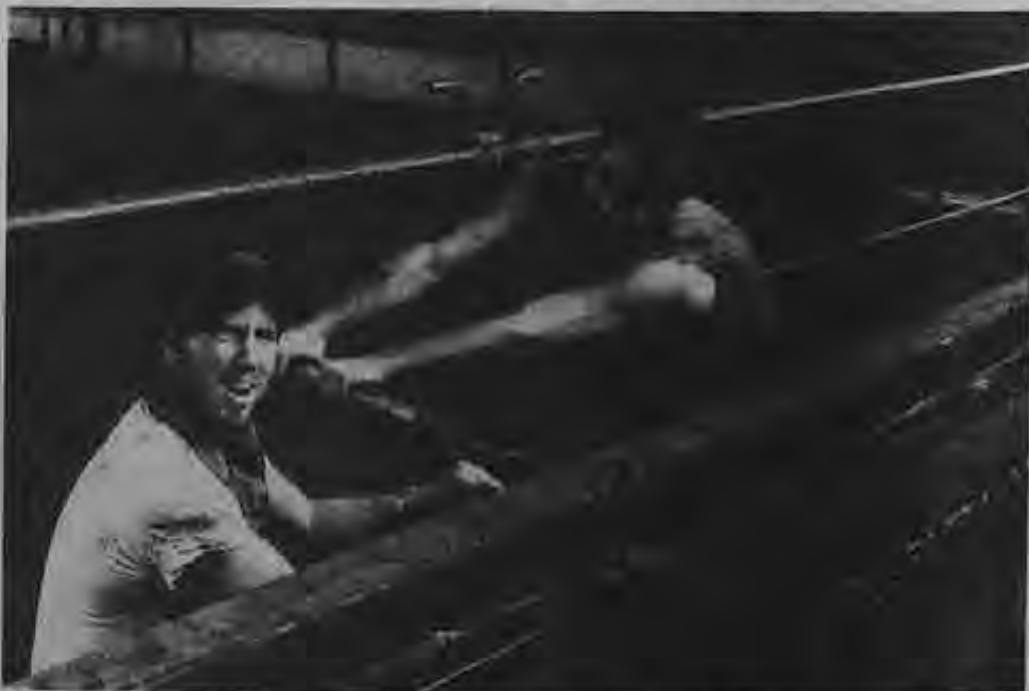
Doing some maintenance work on the crane track are (l. to r.) Dan Gore and Ira Dubson on the Stonewall Jackson .
