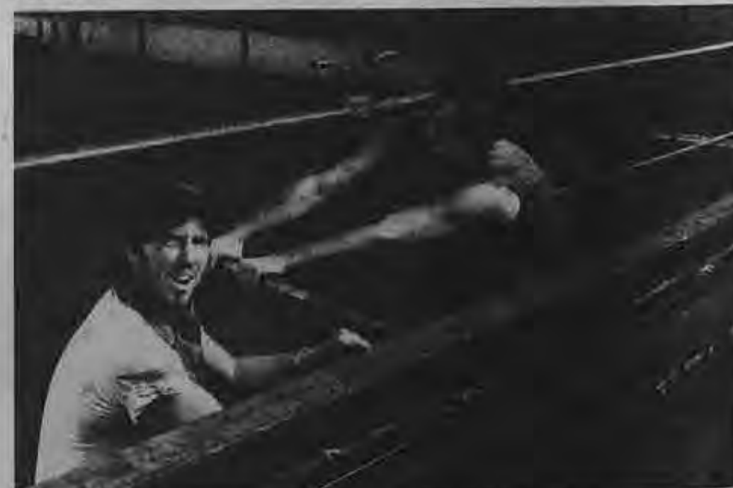
Doing some maintenance work on the crane track are (l. to r.) Dan Gore and Ira Dubson on the Stonewall Jackson .
