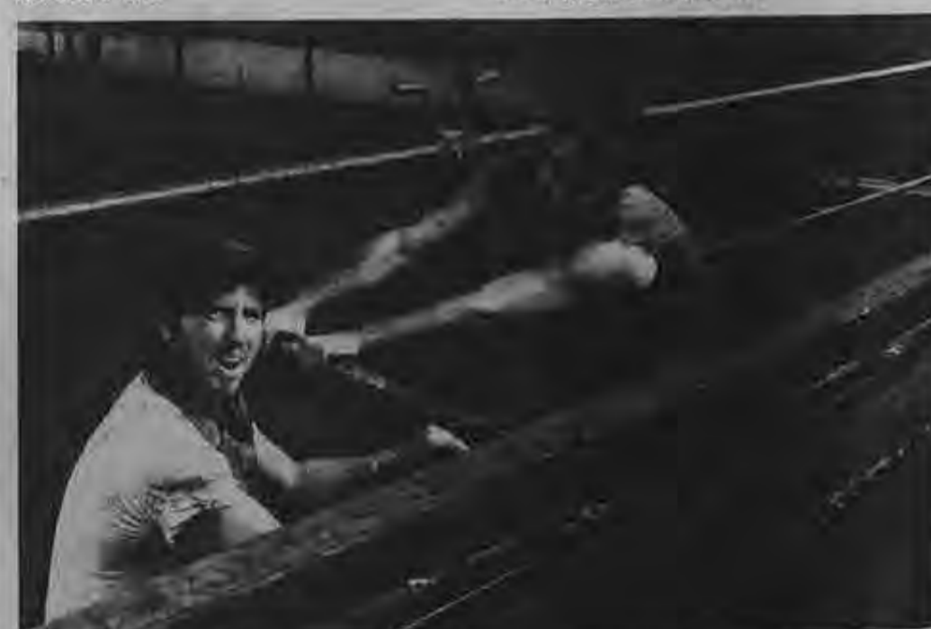
Doing some maintenance work on the crane track are (l. to r.) Dan Gore and Ira Dubson on the Stonewall Jackson .
