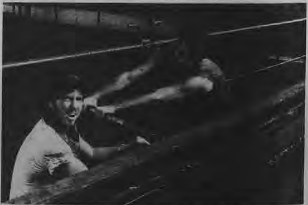
Doing some maintenance work on the crane track are (l. to r.) Dan Gore and Ira Dubson on the Stonewall Jackson .
