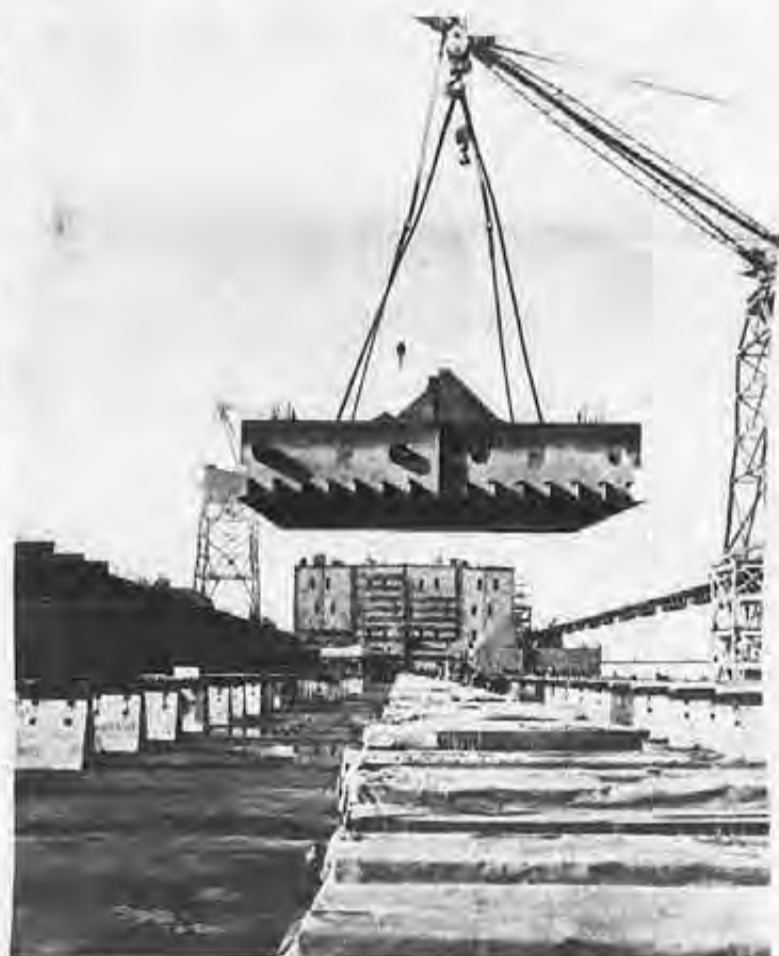
A ship may be under construction in Sparrows Point, Md., as the one above, but pre-fabricated steel and so many other products and supplies needed to build ships come from towns and cities far removed from the yard itself.
