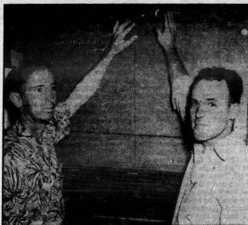
B. B. Tippins, baker, (left) and Patrolman E. B. McAuley, get real close to the new air conditioning equipment installed in the Savannah Hall, which was welcomed by Seafarers who had been sweltering in the Savannah heat.
