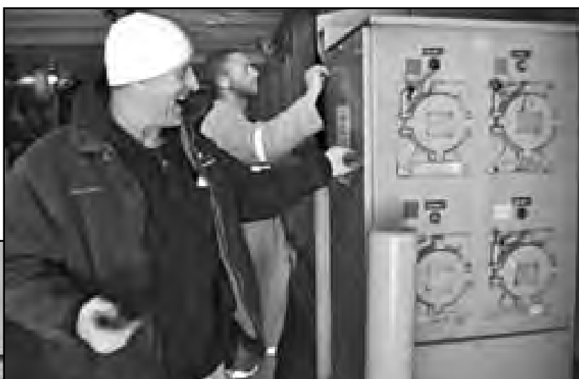
Electrician Bobby Scott (foreground) and Electrician Apprentice Sean Branch put cover on shore power aboard the Antares .
