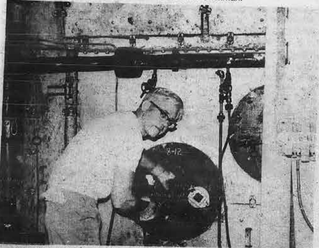
Fireman-Watertender Duane Peterson changes burners in the boiler.
