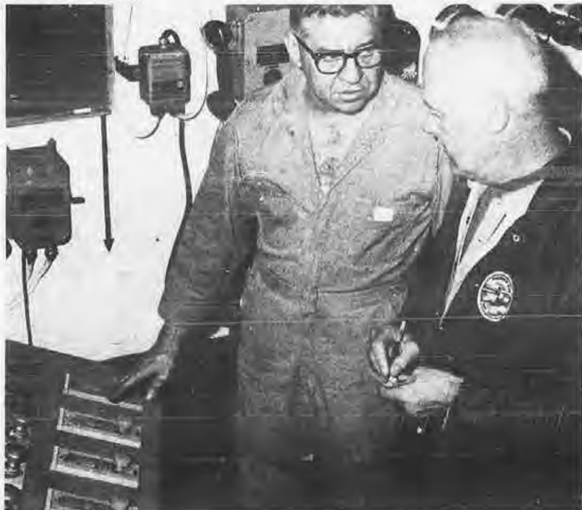
Rex Kauer, oiler (l) explains the operation of the Iglehart's automated console to SIU rep, John McClinton. The Iglehart , a steam turbine, oil burner, had her boilers automated in 1975.
