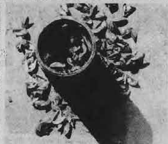
Pictured above are zebra mussels clustered in a water pipe. The mollusks rapidly build up—layer after layer—clogging water intake systems.
