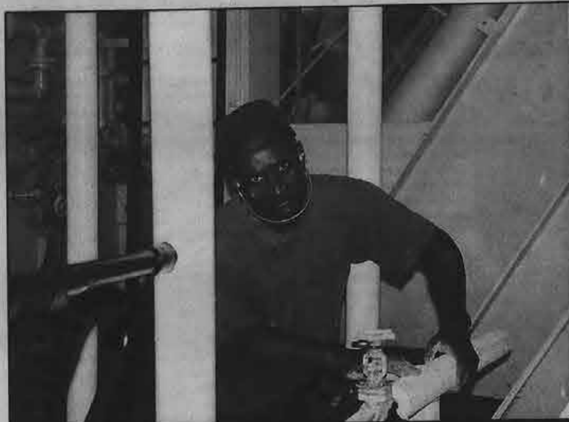
QMED Marcus Hill at work in the LNG Gemini's engine room.
