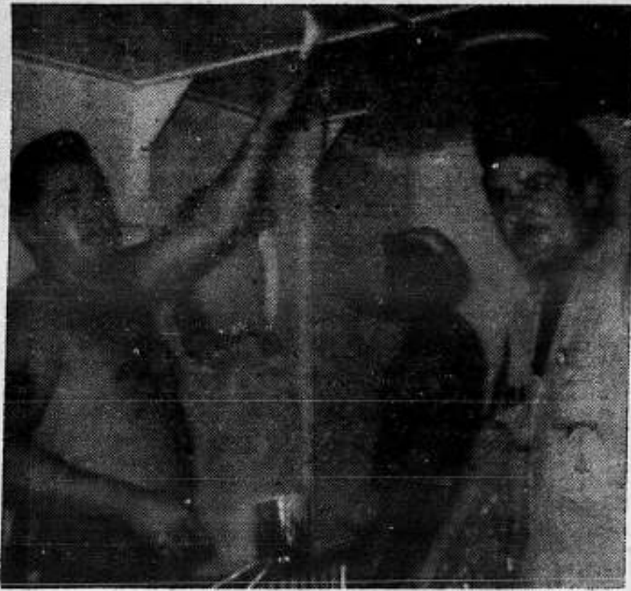
The Western Farmer's recreation room gets a new skin of paint under the careful artisanship of Bosun J. Allen (left) and his two worthy aides, A. Brocato, Deck Maintenance, and J. Burg, AB. The hard working deck gang transformed the Farmer from a rusty ex-boneyard scow to a trim-looking ship in a few weeks, photographer Gowder reported.
