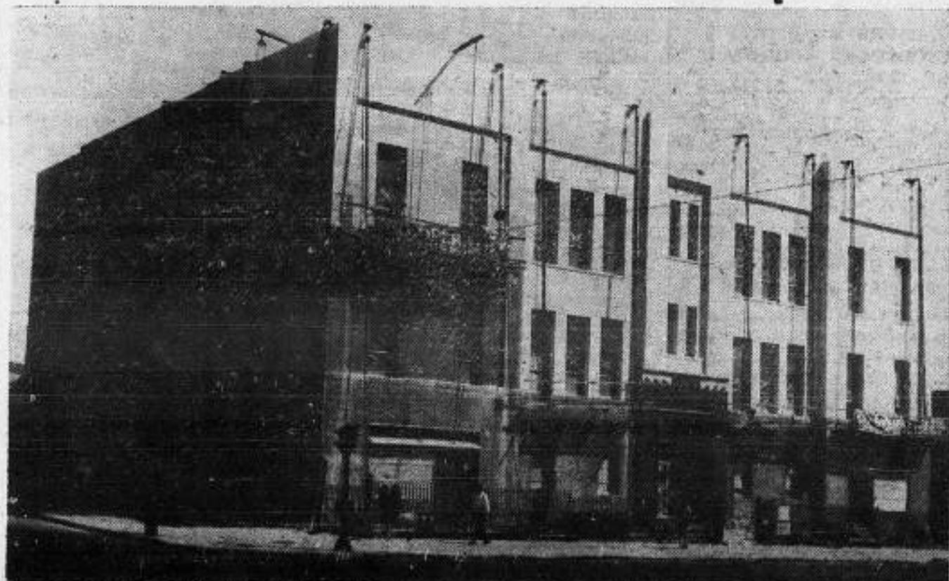
The new Headquarters-New York Branch building nears the end of its face lifting in the front. When the picture was taken workmen were completing the application of simulated white limestone to the upper two stories and were readying work on the brownstone to be put on the front of the first story.
