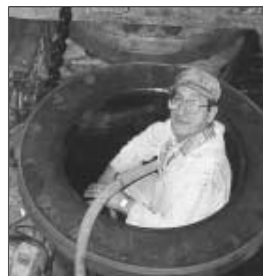
Right: DEU Dave Mathes cleans the cylinder on the Southdown Challenger's main engine.
