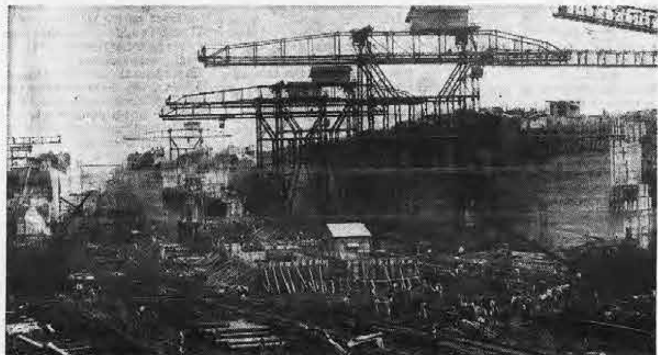
Workmen are dwarfed by huge concrete structures rising in the Miraflores locks, as builders slice through massive hills. The scene is looking north from west bank on August 16, 1912.
