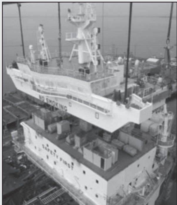
A final piece of the first tanker of five new builds for APT is lowered into place at General Dynamics NASSCO.
