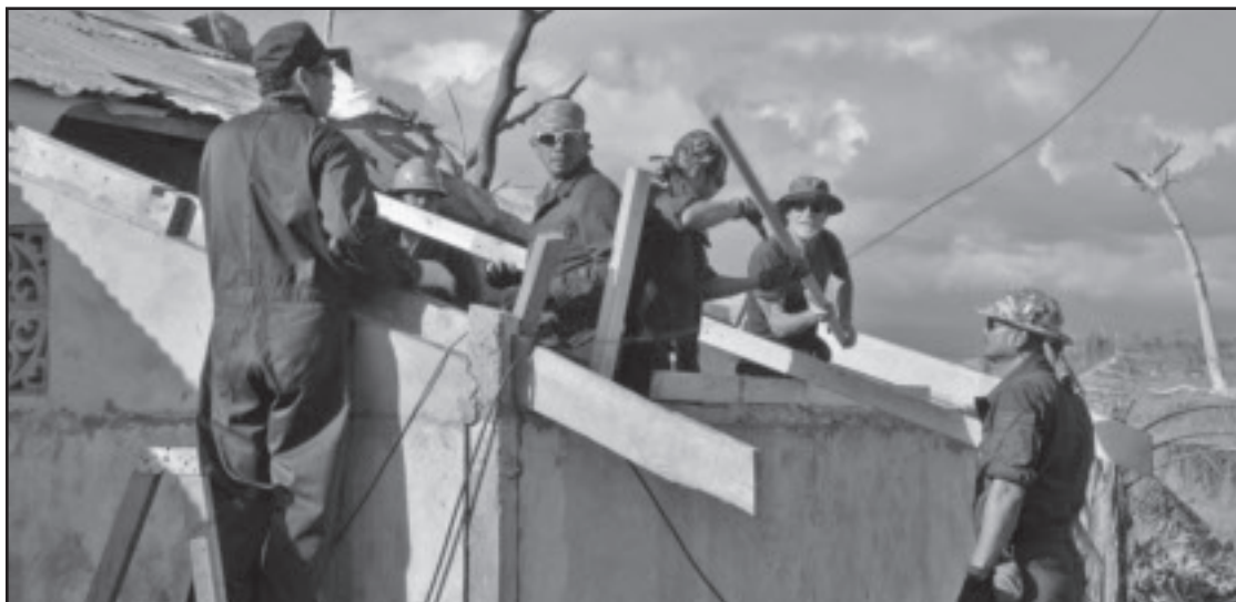
Mariners from the SIU-crewed USNS Charles Drew repair a roof in the Philippines following the devastation brought to the region by Typhoon Haiyan. (U.S. Navy photo)
