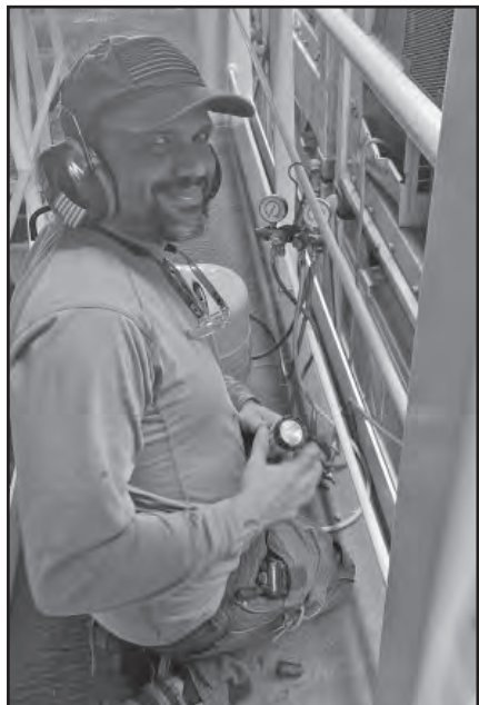
Electrician Carlos Parrilla handles maintenance on a reefer container aboard the Taino .
