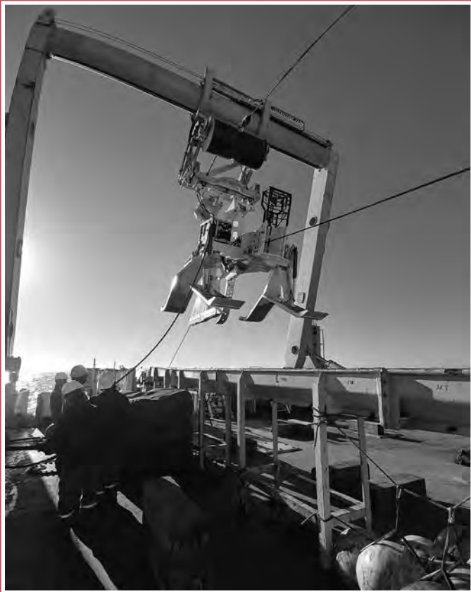
Crewmembers aboard the CS Decisive (photo above) prepare to bury cable using a device called a Plough. In addition to burying the cable two meters under the ocean floor, the mechanism also lays the cable. In the photo at immediate right, a vessel hauls shore end cable to the beach where ultimately it will be connected to a shore side station. Thanks to Recertified Bosun Victor Nunez for providing these photos.
