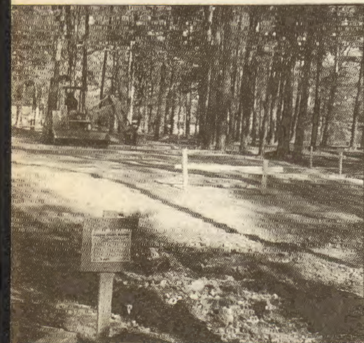
Groundbreaking for the new simulator classrooms at the Paul Hall Center took place last month.
