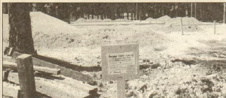
Construction continues on the new Paul Hall Center building that will house simulators for shiphandling, engine room operations, crane operations and liquid cargo procedures.
